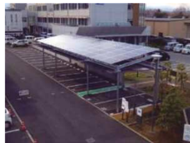
Solar carport at Hachioji Water Supply Office
