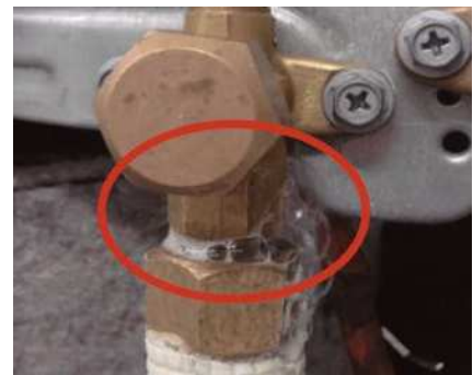
Leakage of fluorocarbons
