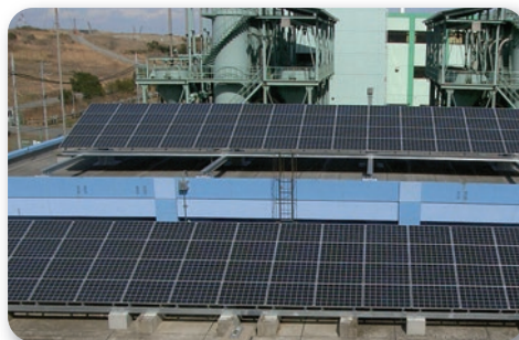
Solar power generation system
