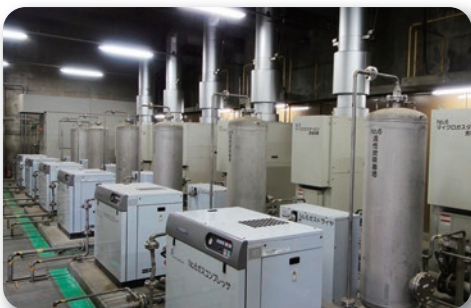
Landfill-gas utilization facility with micro gas turbines
