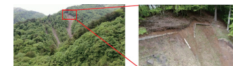
A distant view of a collapsed area (Photo taken by a drone)
